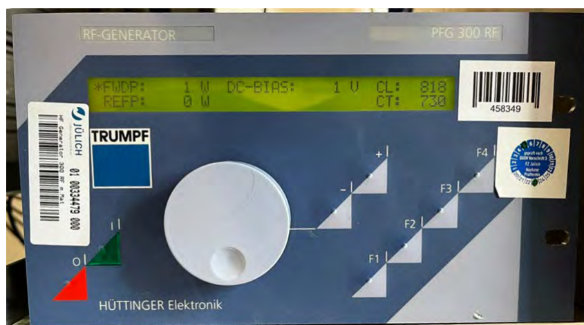
Figure A.22.: RF generator panel.
