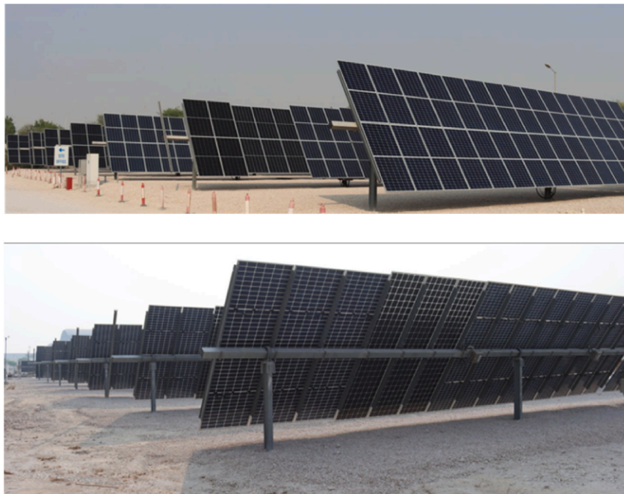
Fig. 1. Photographs of the front (top) and rear (bottom) of the Horizontal Single Axis (HSAT) testbed installed at the outdoor test facility (Doha, Qatar). Trackers 2, 4, and 6, each consisting of eight strings, will be the focus of this study.
