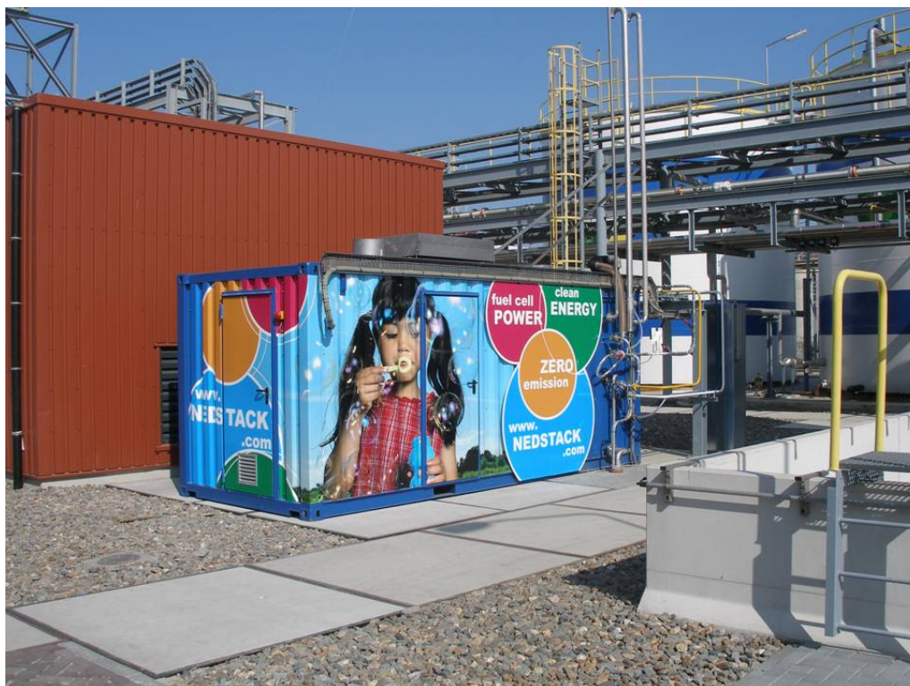
Figure 2: Container with the 50 kW PEM Power unit at the Akzo Nobel chlor-alkali plant in Delfzijl.
