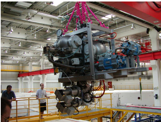
Fig. 1: ABS and supporting bridge with suspension frame in flight to the ANKE target place. The main designer (F.K.) stands below in the opened COSY tunnel, trusting his constructions.
