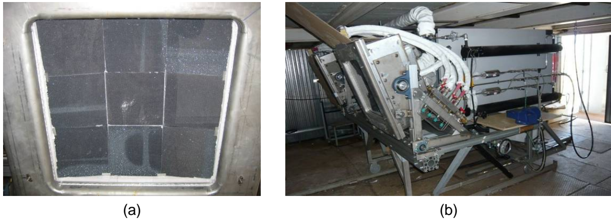
Figure 1: Pilot, 100 kW-scale HYDROSOL solar reactor: (a) front face of reactor's individual chamber consisting of nine SiC square-shaped blocks; (b) dual chamber reactor completely assembled and installed at the SSPS tower, ready for operation.
