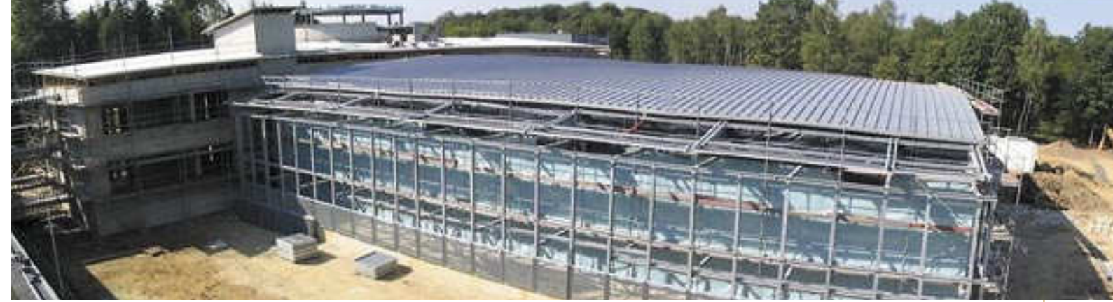
Figure 2: View of the new machine room in Jülich, being built for the IBM supercomputer
