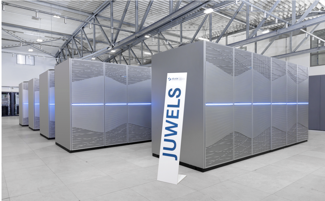
Figure 1: The Cluster Module of the supercomputer JUWELS in the facility of Jülich Supercomputing Centre. Copyright: Forschungszentrum Jülich GmbH.
